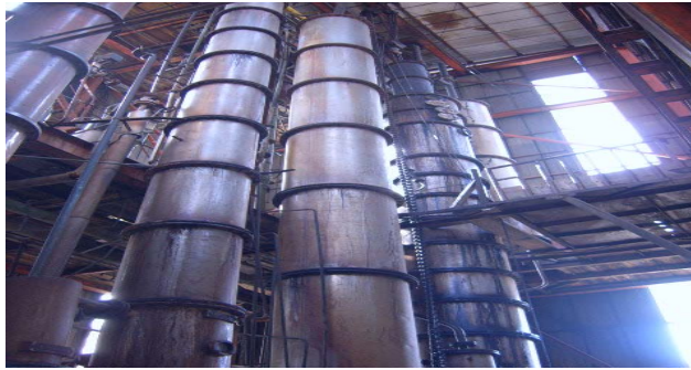
Fig 5.3 Factory Distillery Columns
