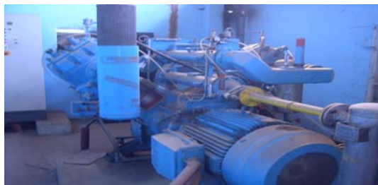
Fig 5.2 Factory Air Compressor
